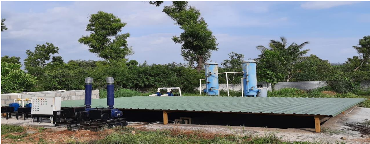
Figure: Waste water Treatment plant located at ATME campus
